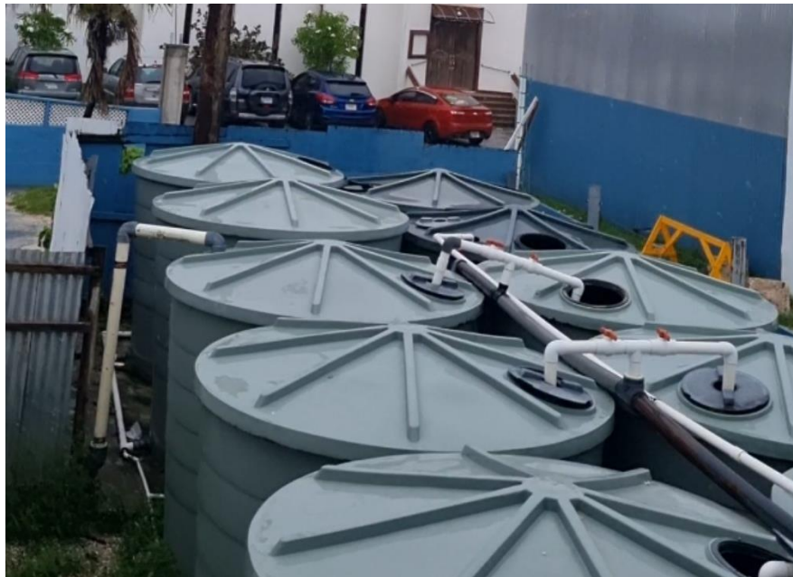
Plate 4: Water tanks (12 pcs) at the CMI site
